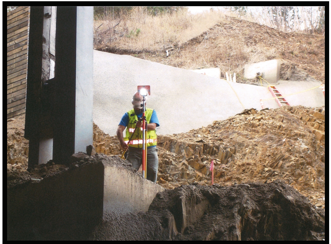
Jason Dahlman (CETEC Engineering) monitoring piles for movement during excavation. In the background are excavation and soil remediation for location of the future hotel. Smart targets on pile caps were installed for accuracy and convenience.
