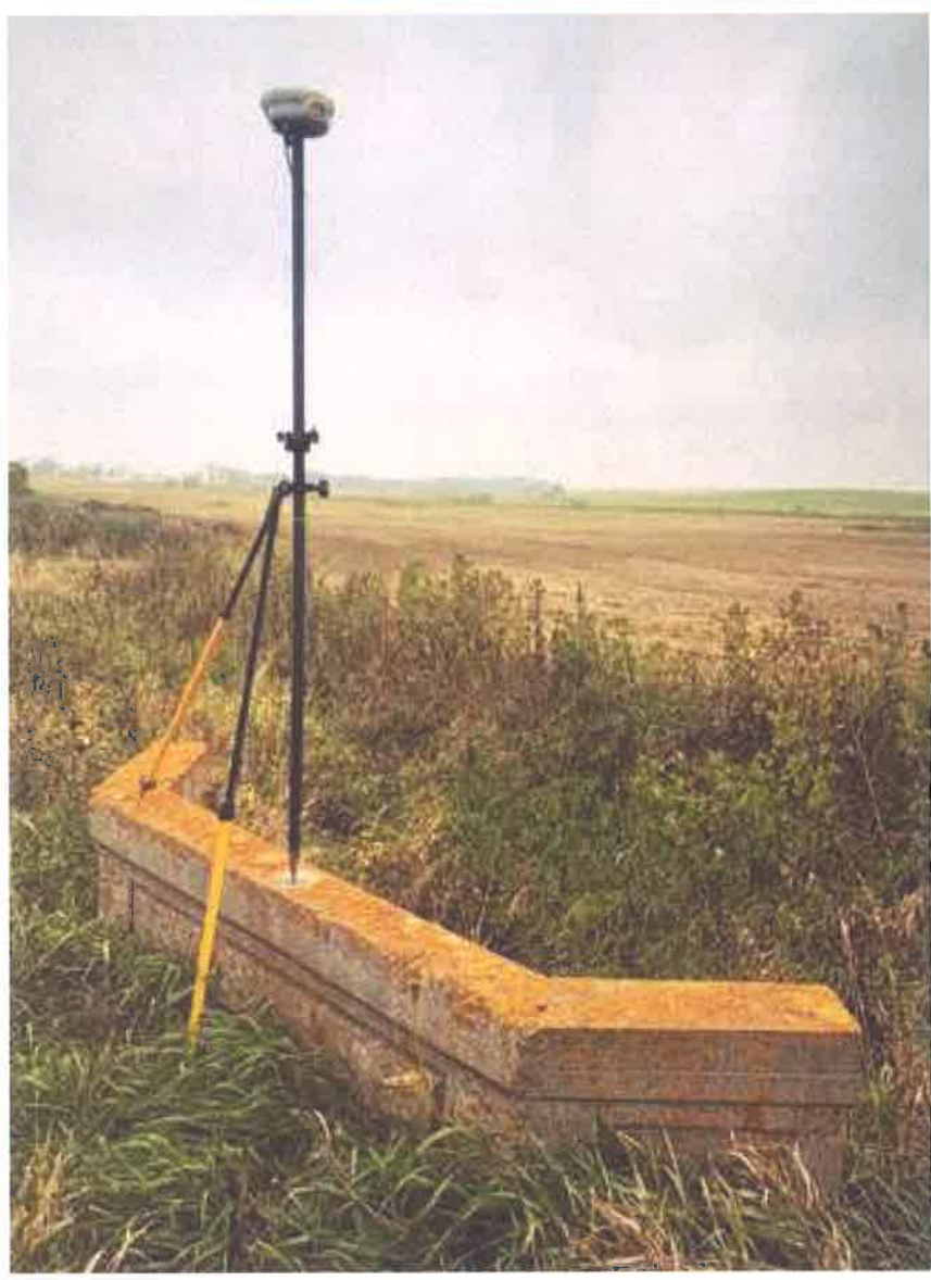
N62 Disk in Old Culvert Headwall on Old SD Hwy 10 3.3 Miles E of Lake City, SD
